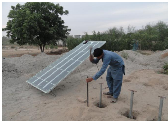
Figure2. Alignment of poles for solar desalination mounted on pole
