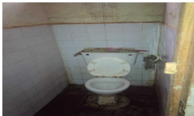
Figure6. The condition of public latrine at Post Office Akure, Ondo state
