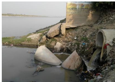
Photo8. Confluence point of Tefco Nalla having partly tapped
