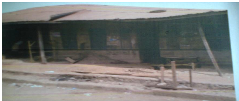
PLATE 4.2 Sustainable dilapidated Building at Osupa, Ogbomoso
