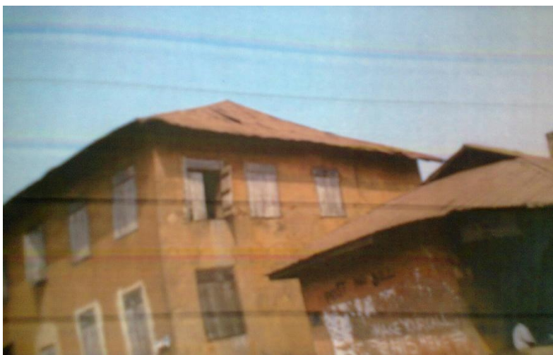
PLATE 4.3 Building with Timber Panel Window and No Anti Burglary Grilles at Jagun, Ogbomoso
