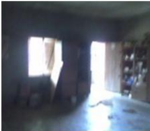
Broken walls into classrooms
