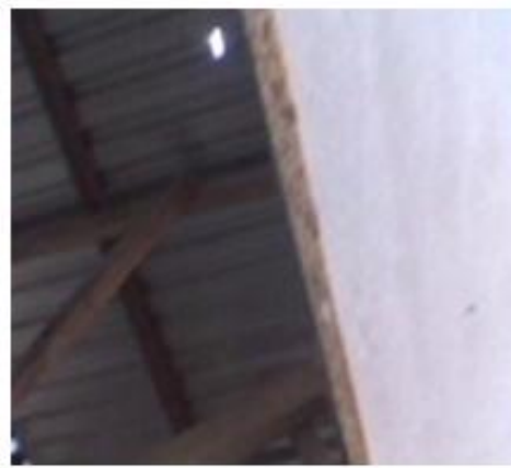
Dilapidated roof classroom building in use
