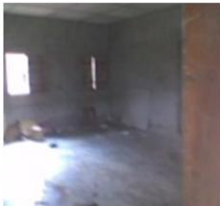
Broken walls into science laboratory
