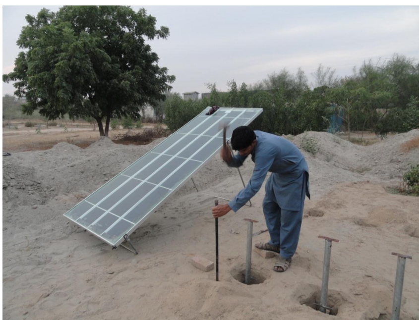
Alignment of poles for solar desalination mounted on pole
