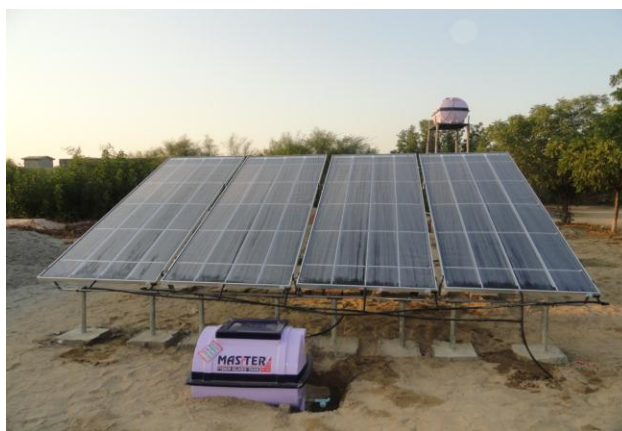
Four unit of solar desalination installed at AZRI, Umerkot, Sindh
